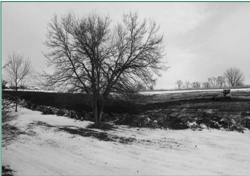
Work begins on the future site of the solar panels that will power Clare House at Mount St. Francis Center.
